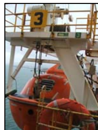
Existing Lifeboat Installation
