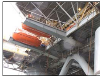
Existing Lifeboat Installation
